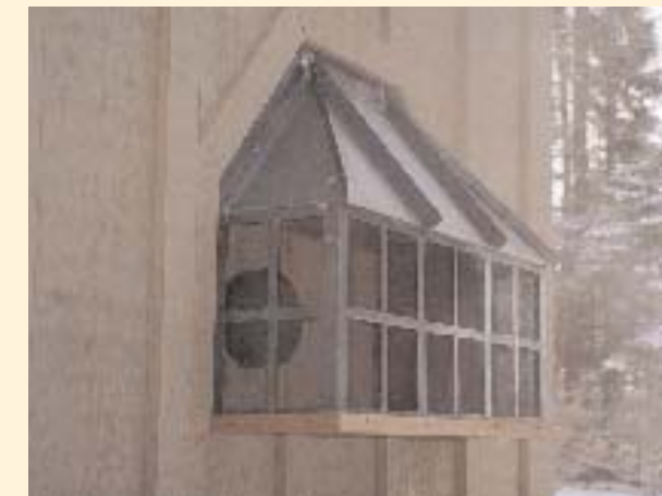
Creative deception. Designed to resemble Craftsman-style light fixtures, a custom-built cover conceals the heating system's intake and exhaust pipes. Photo taken at F on floor plan.
